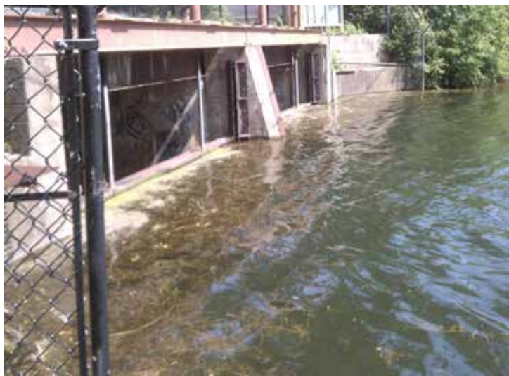
Outlet gates in the closed position
