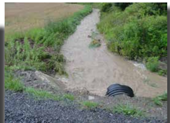
Undersized culvert caused substantial road bank flooding and re-routing of water.
