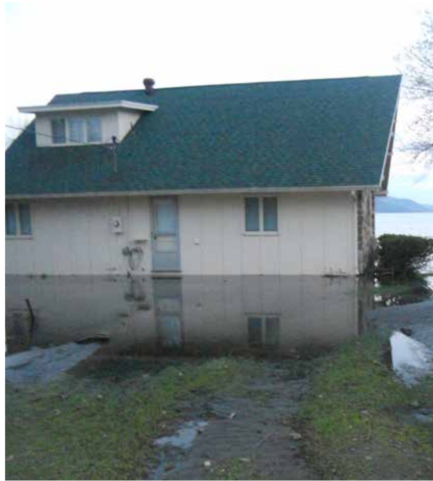
Lake water flooding a low lying home during the floods of 2011.
