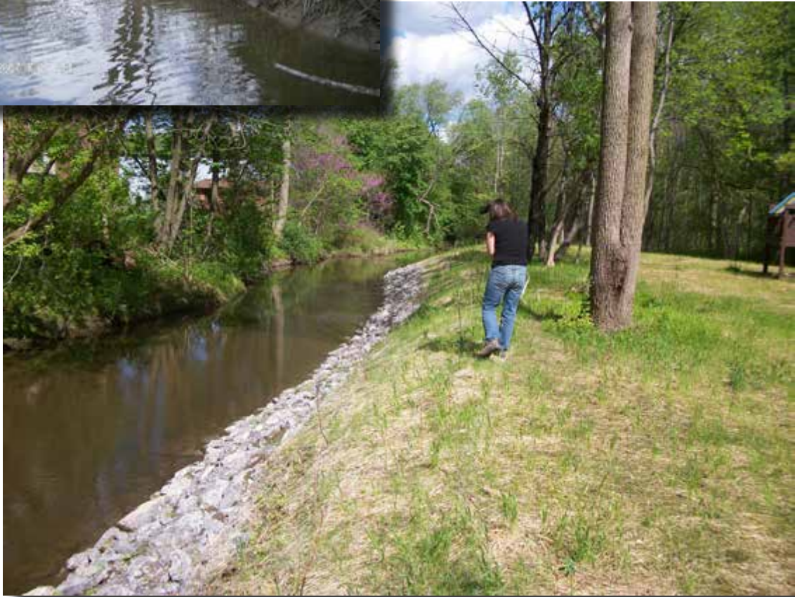
Project along Sucker Brook- project completed with the Town of Canandaigua installing toe stone protection and plantings on the upper two thirds of the creek.
