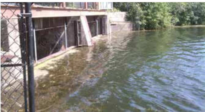
Outlet gates , located behind Wegmans, in the closed position
