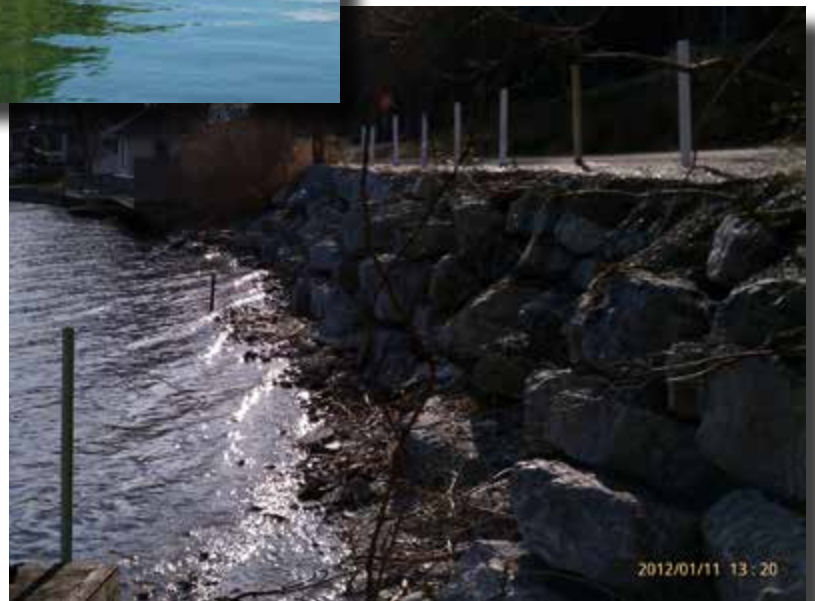
Rock stabilization along an existing road was the only solution after the floods of 2011.
