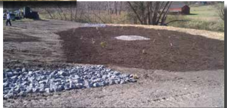
Middlesex Highway Department Bio-retention Area
