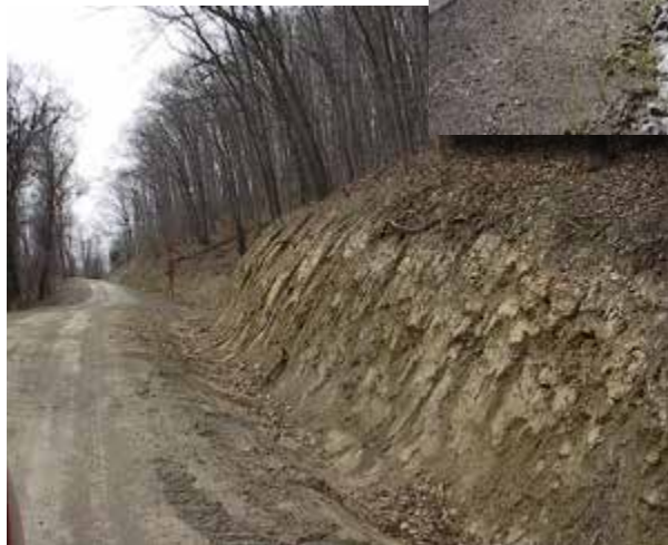
Potential for major roadbank erosion.
