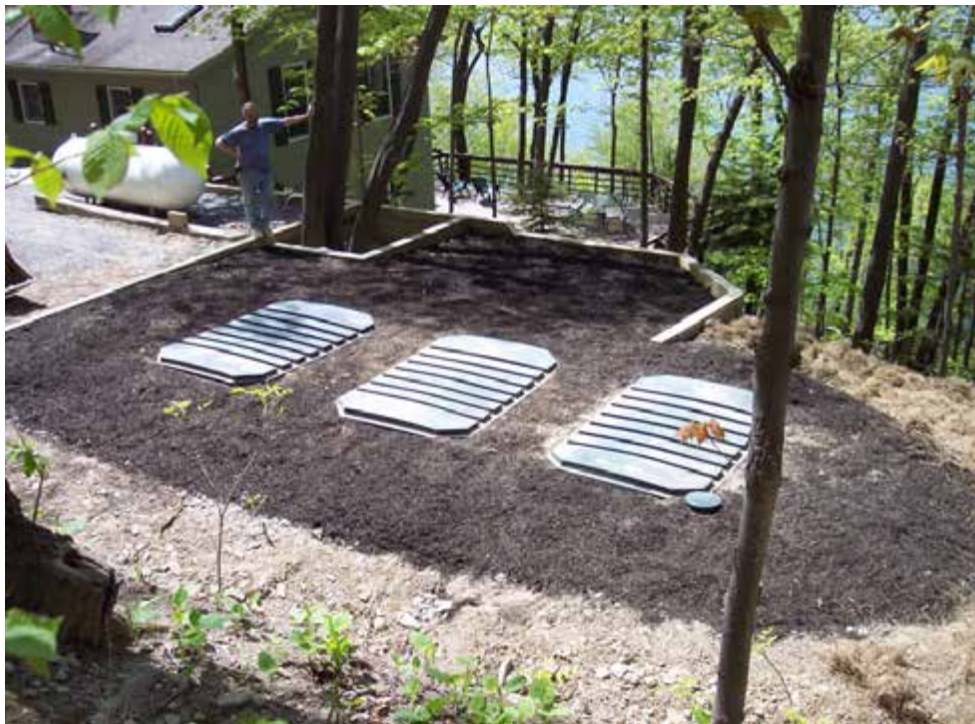
Peat moss alternative septic system.
