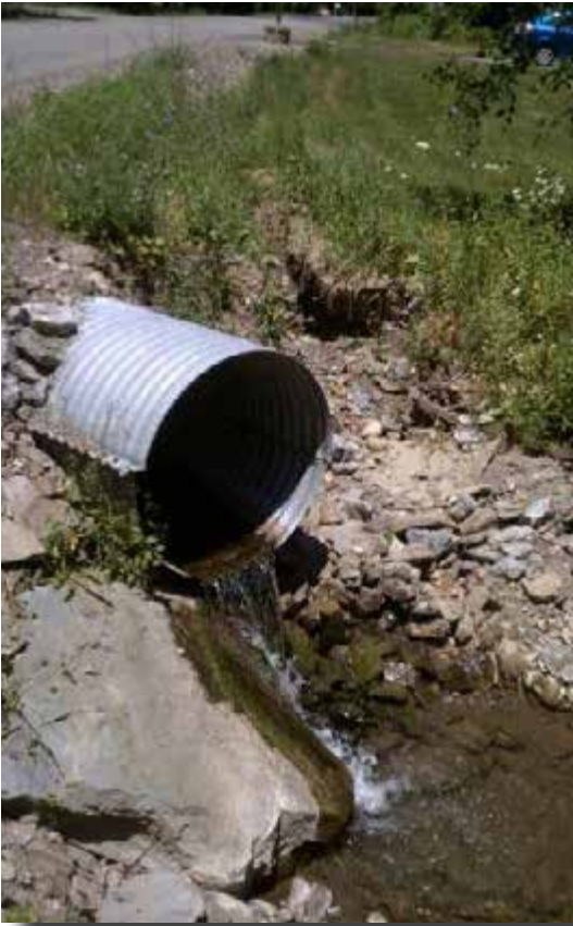
Undersized and difficult for fish passage- needs to be embedded.
